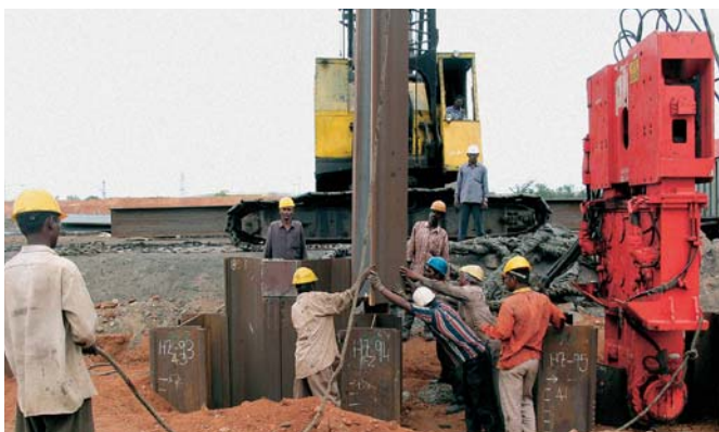
Due to the presence of weathered rock an impact hammer was needed to fully drive the sheet piles
