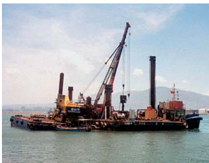
Two cranes, an ICE vibratory hammer and an impact hammer made up the installation equipment
