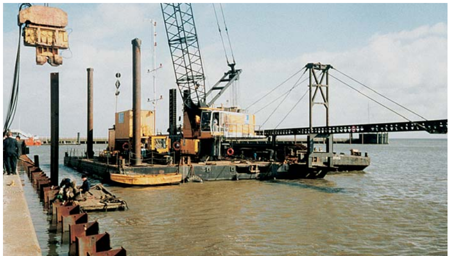
After installation of all the king piles, the AZ sheet piles were driven to El. -20 m
