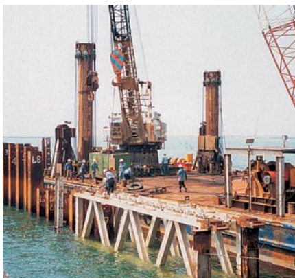
Driving was occasionally executed below the waterline because of substantial tidal variations
