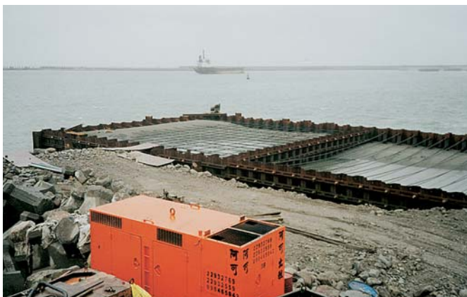
The 27.4-m return wall of Quay 15 consists of a combined wall with 14 HZ king piles
