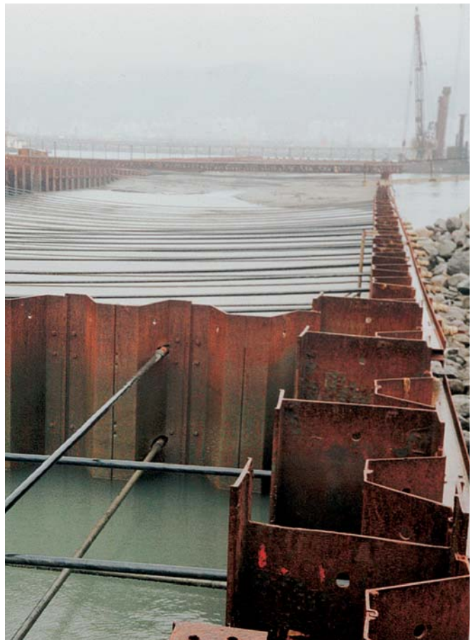
Numbers of tie rods cross over each other to connect the main and return walls to their respective anchor walls
