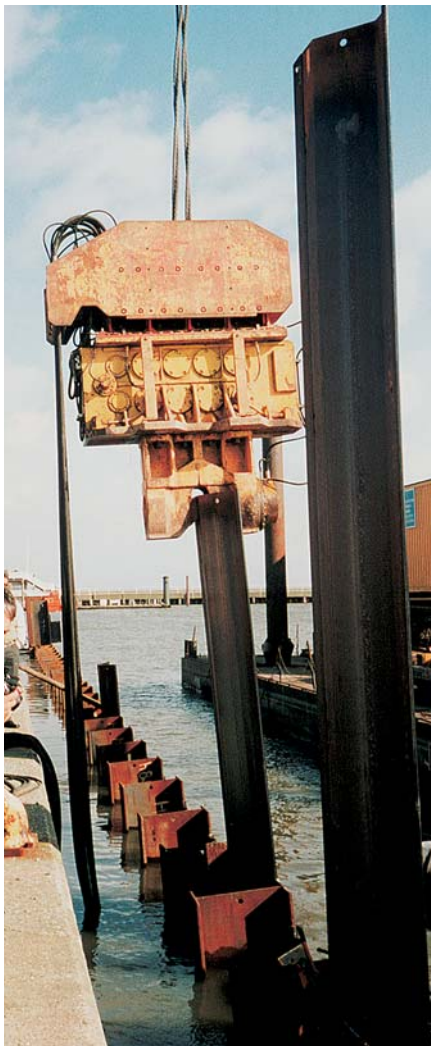
The vibratory hammer was the ideal tool to install the AZ intermediary sheet piles
