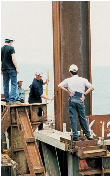
Two engineers from Arcelor were dispatched to the site for assistance during the installation process
