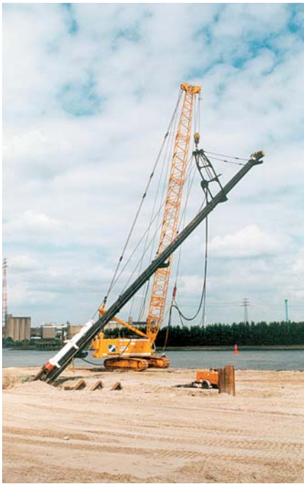
The 47-m tailor-made HTM 600/136 anchor piles were driven with a hydraulic impact hammer
