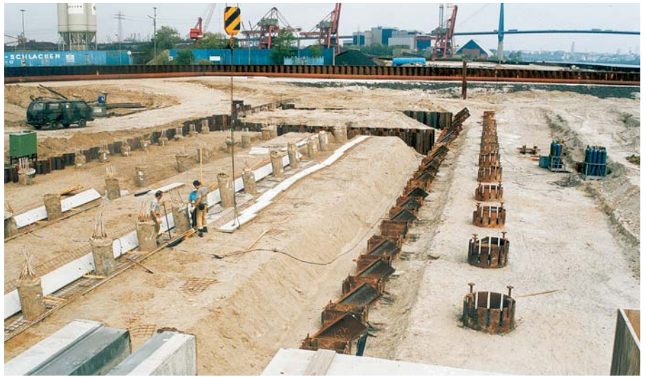
The low-level superstructure slab is placed on top of the two sheet pile walls, steel tension piles, fender tubes & concrete piles
