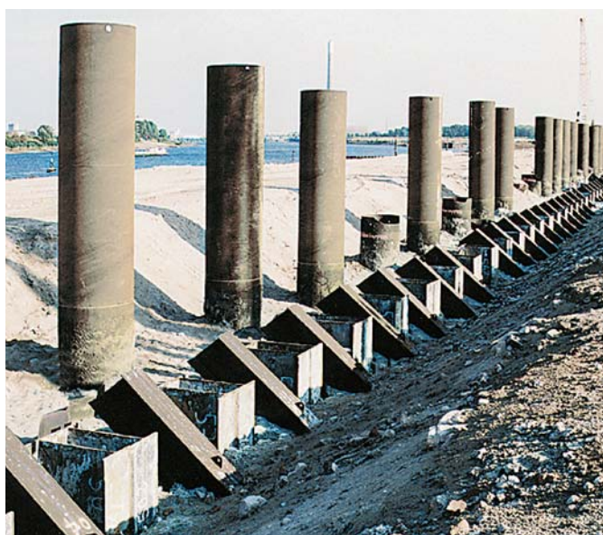
Tubes placed in front of the sheet pile wall act as fenders
