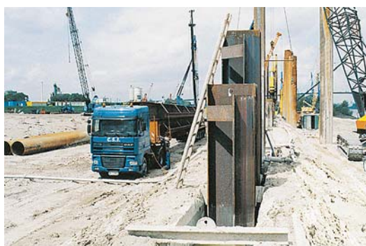
Due to difficult soil conditions, and as a means of reducing vibration, the sheet piles were driven in a bentonite-supported trench
