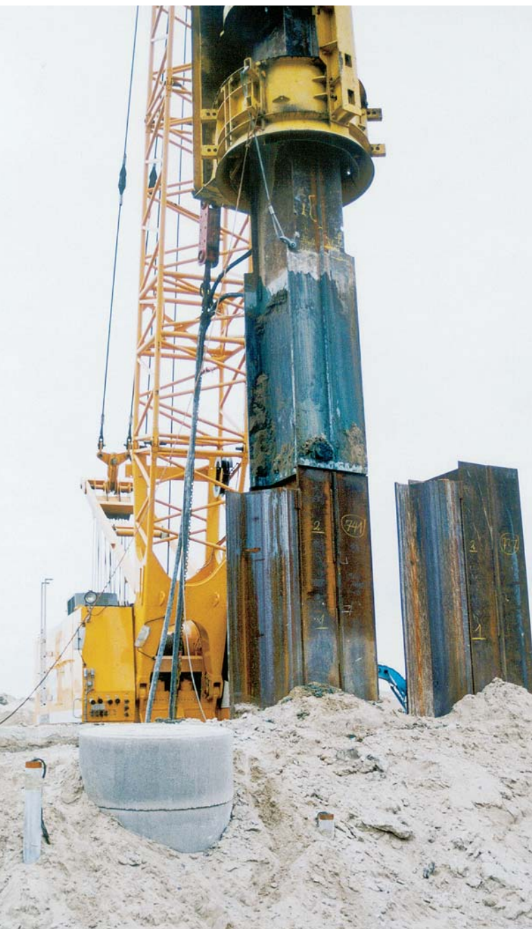
The heavy sheet pile elements were driven to a depth of 30.5 m with an impact hammer
