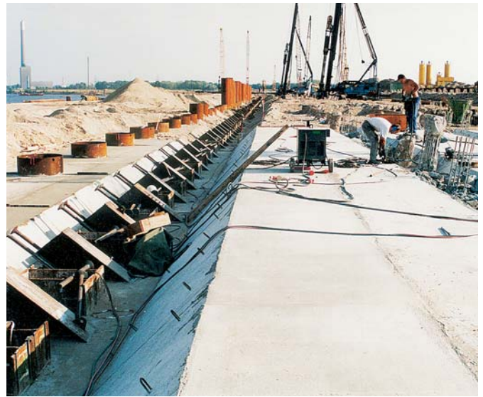
After pouring, the concrete of the relieving platform was covered with a 3.3 m sand layer
